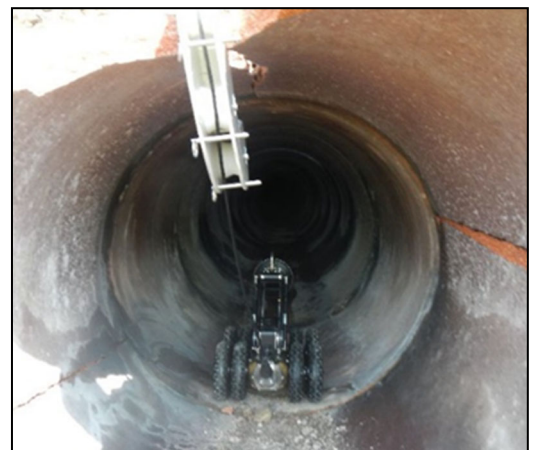
(top) Removal/decontamination of sewers, underground foundations at the former SFAAP. (bottom) Robotic crawler inspects pipe.
