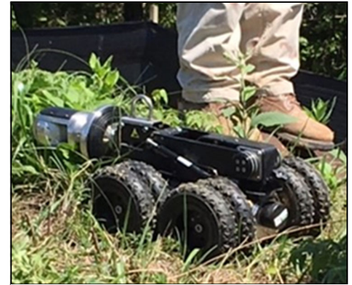
USAE's Pearpoint flexitrax 350 robot being prepared to visually inspect a section of 36" diameter pipe
